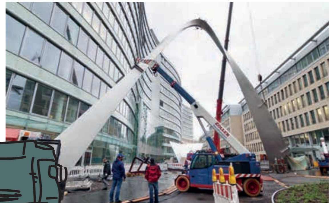
That was real precision work: semitrailer trucks transporting giant arches for an aluminum sculpture for the Frankfurt office complex “The Wave,” where they were welded together, erected, and assembled | Image: M. Pyper
